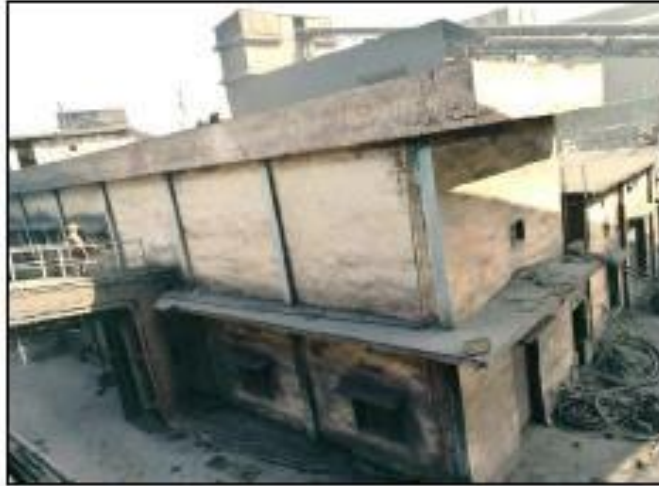
Sponge Iron Control room
