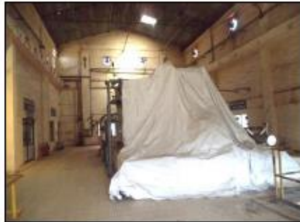
Internal View of captive power plant
