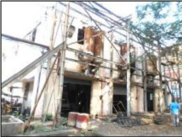
External view of DG Room
